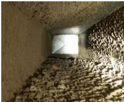
Fig. 1. Air duct accumulated with dust
